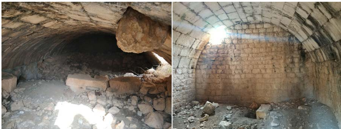
Figure 9. Interior views of underground storages: North storage (left) and south storage (right).
