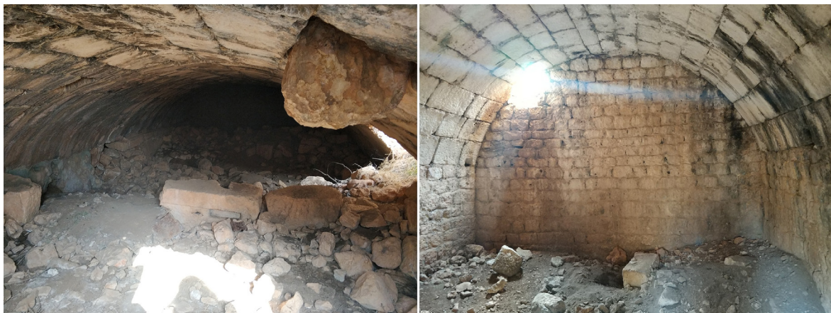
Figure 9. Interior views of underground storages: North storage (left) and south storage (right).
